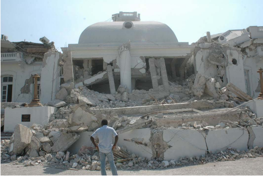
The area below the central dome suffered the worst damage, pictured from the front above and from the rear, below
