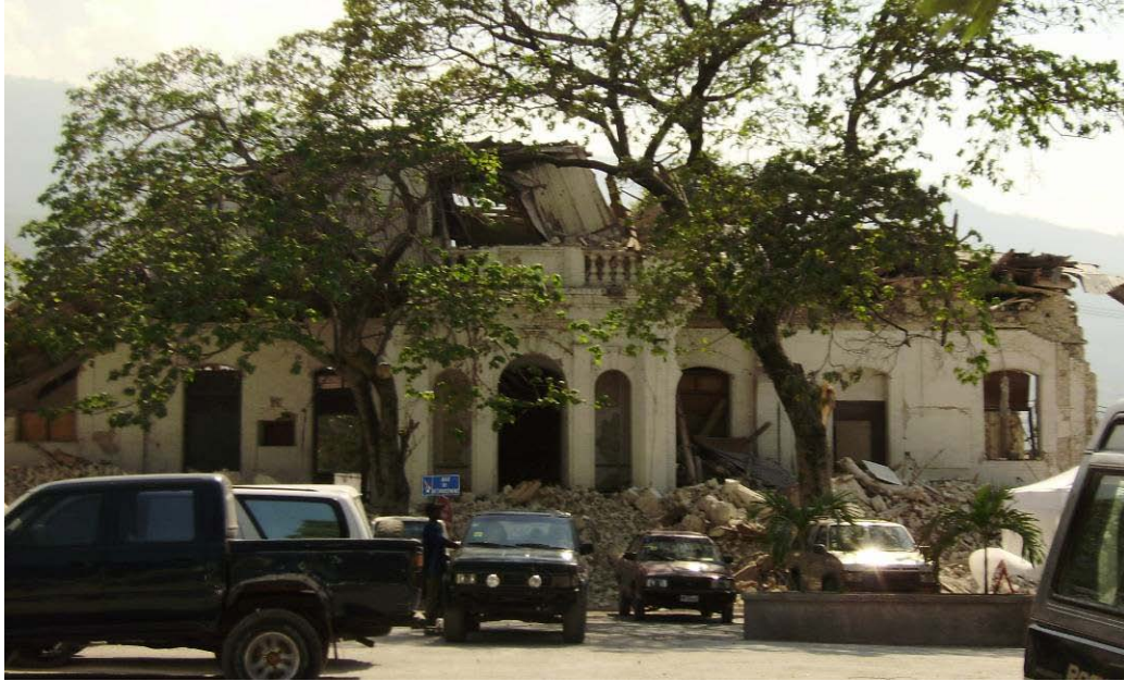
The Casernes, which sits just to the rear (south) of the Palace was severely damaged
